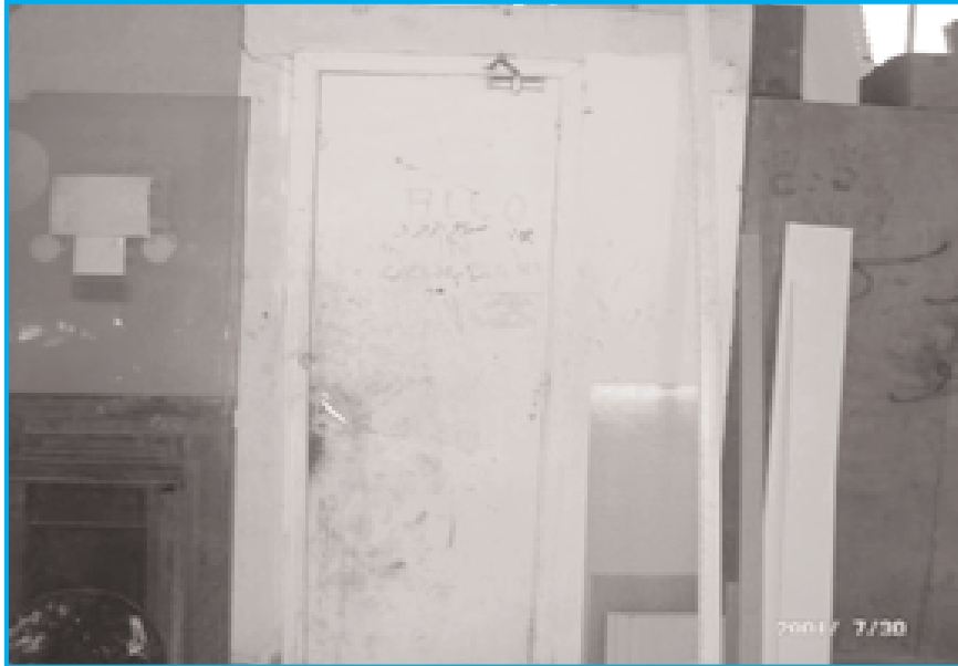
Photo 3: General lavatory hygiene condition unacceptable. (Observe the hygiene conditions of the door to the lavatory. The conditions inside were by no means acceptable).
