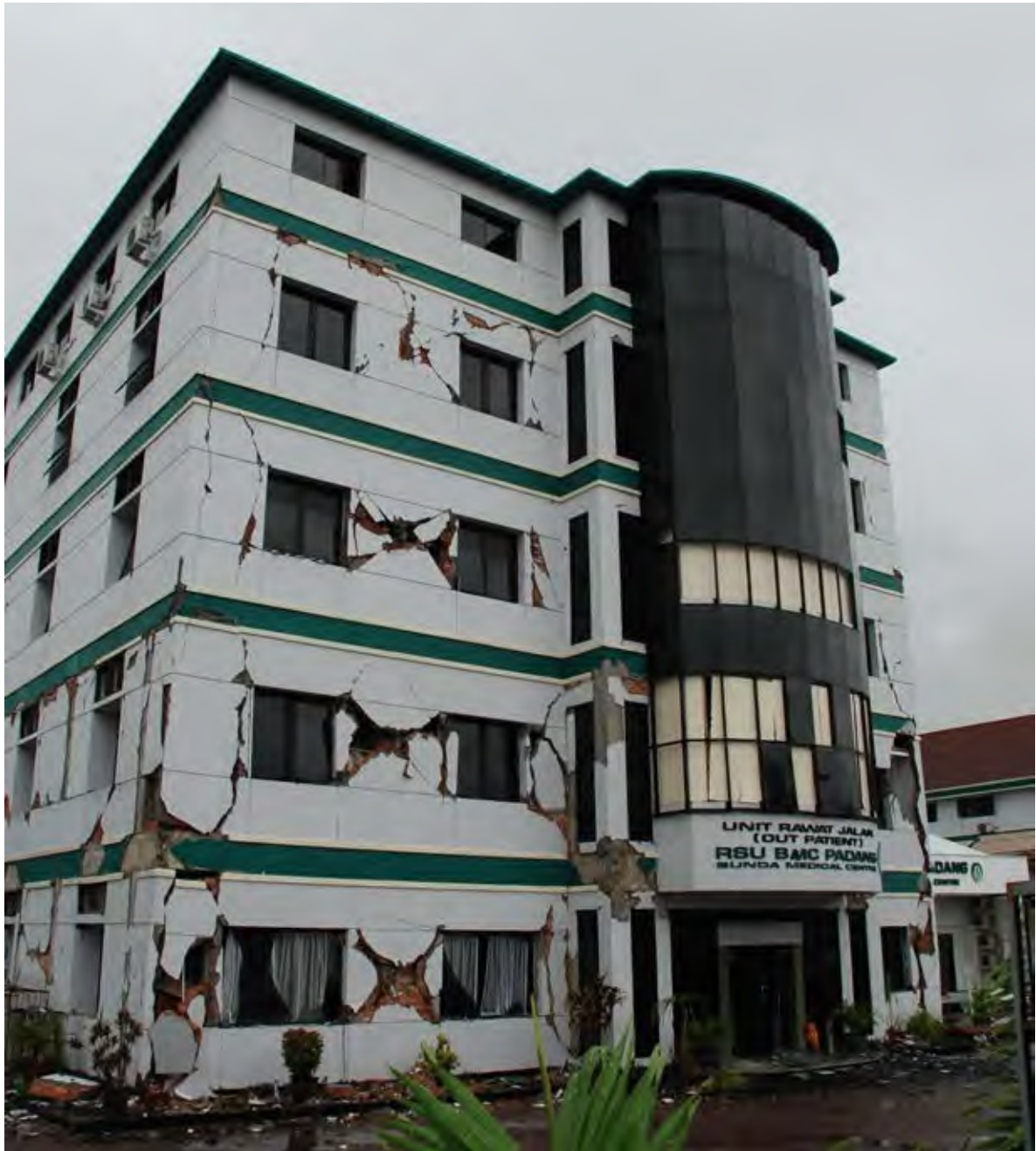
Figure 2.8 Restu Ibu hospital was severely damaged by earthquake in Padang. Source : BNPB
