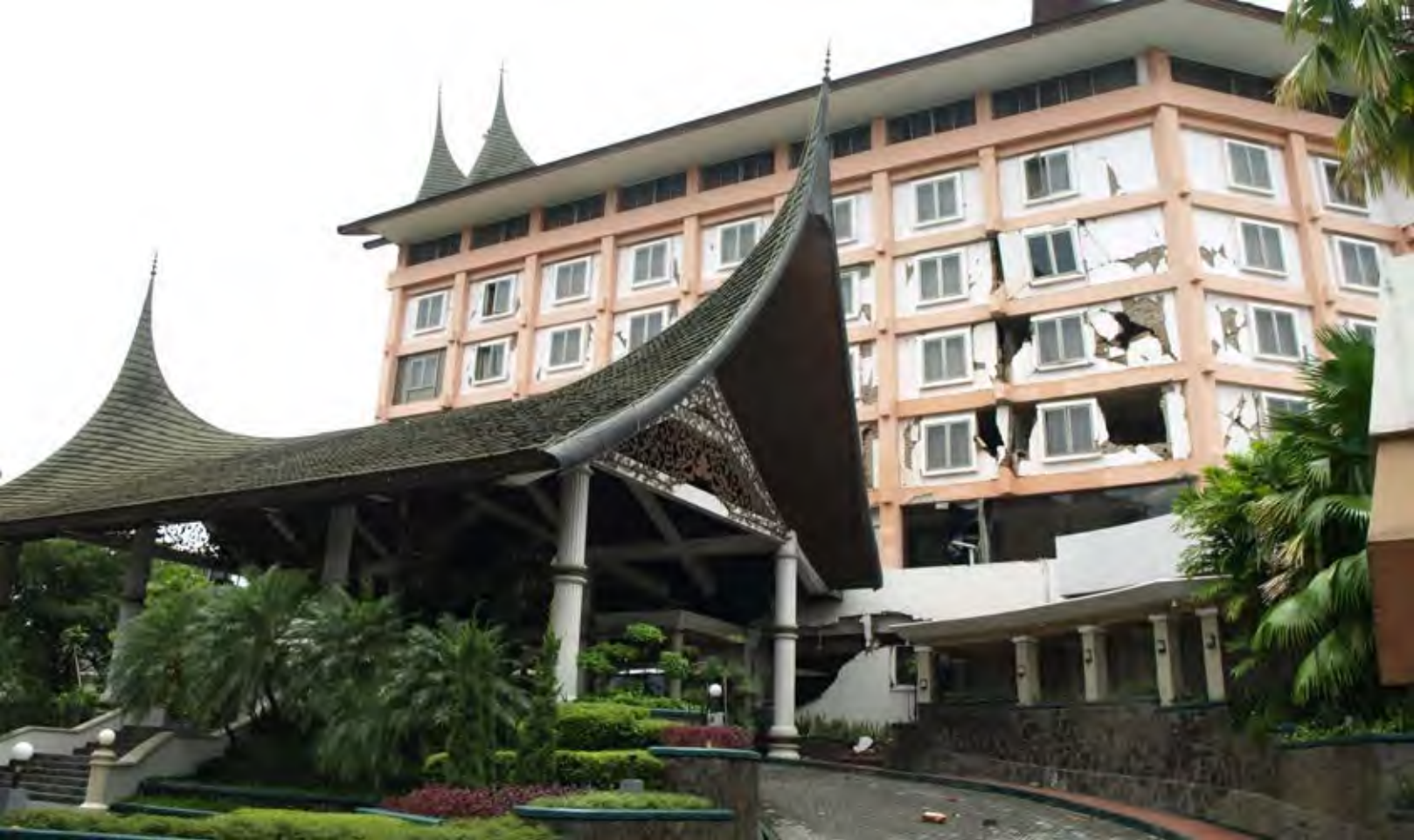
Damage hotel after earthquake in Padang. Source : BNPB
